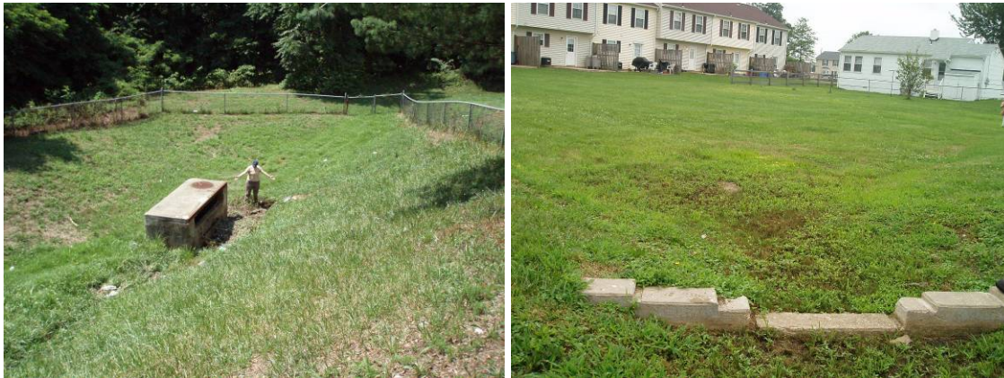
Figure 3-6. Diggs Circle Dry Pond (L). Carroll Street Dry Pond (R).
