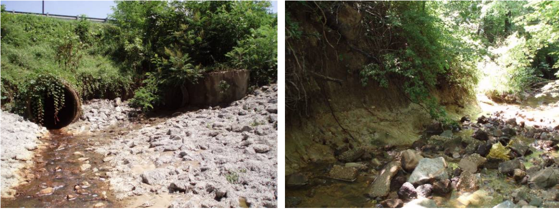
Figure 3-4. Double outfall (L). Scoured downstream channel (R).
