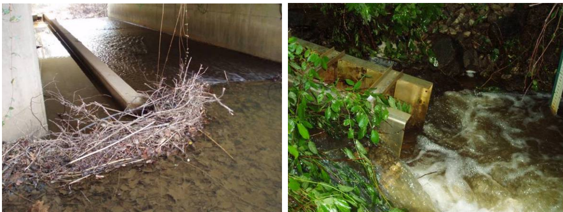
Figure 3-1. Fish Ladder at MD 6. Left – Upstream end. Right – Pool at bottom.
