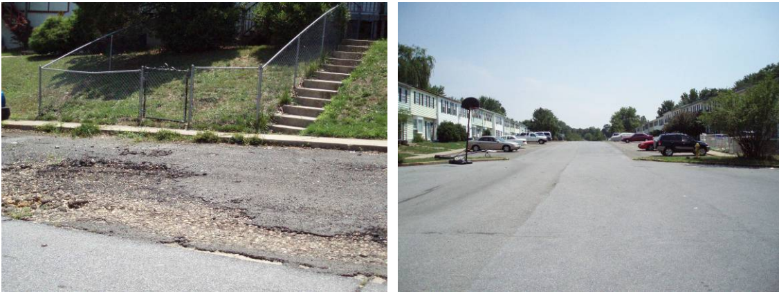
Figure 3-7. Patuxent Court. Asphalt parking spaces in disrepair (L). Configuration of road, parking, and cul-de-sac (R).
