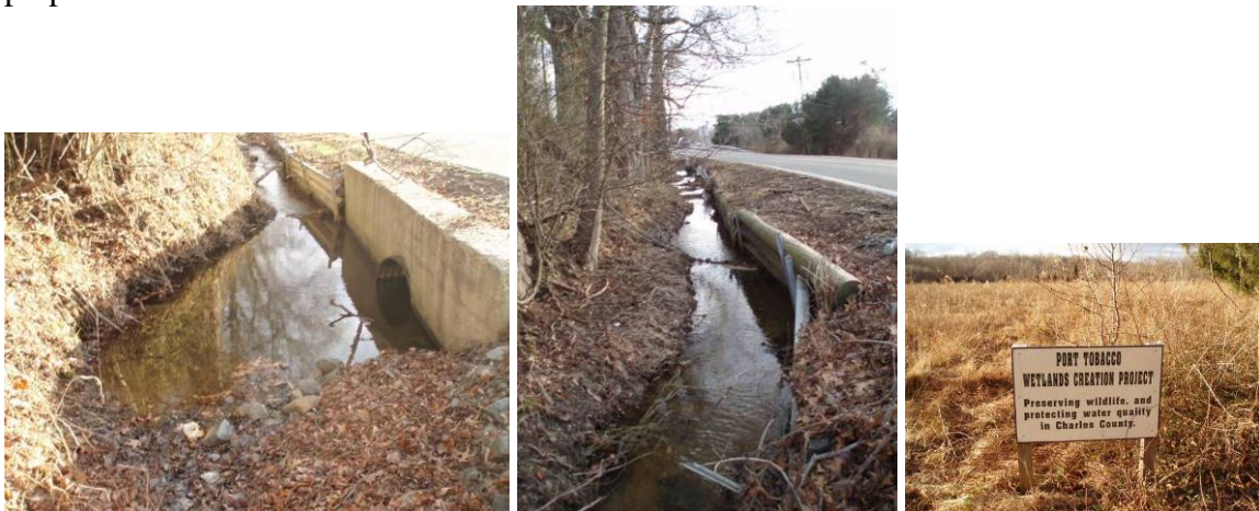
Figure 3-2. Stream Reach 24 along Mitchell Rd. (Left) dysfunctional culvert; (Center) Flow parallel to Mitchell Road; (Right) Commercial wetland mitigation site across Mitchell Road.
