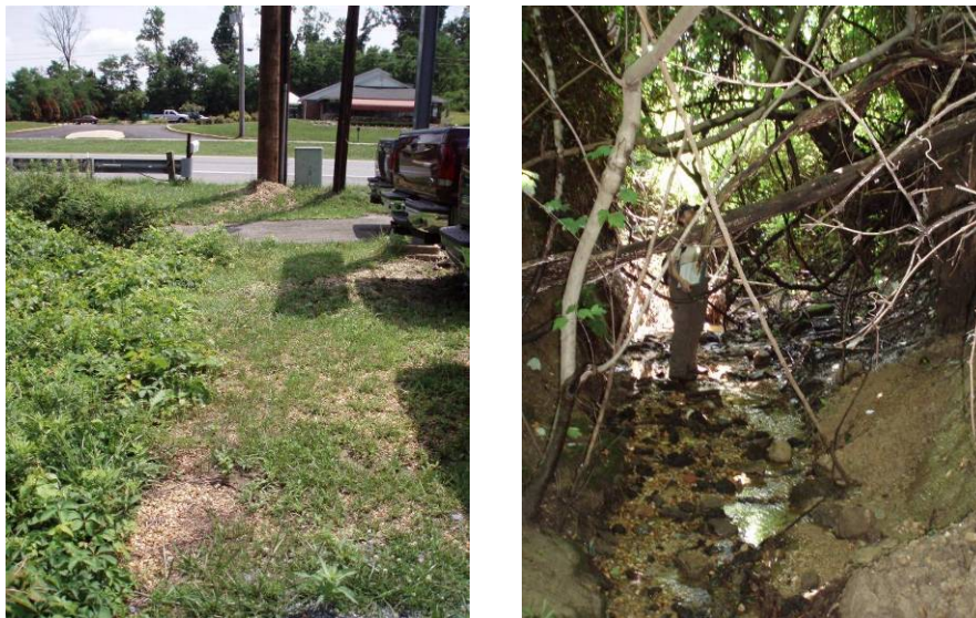
Figure 3-5. Channel adjacent to Hunt Ford. View of concrete chute at top (L). Depth of channel compared to person (R).
