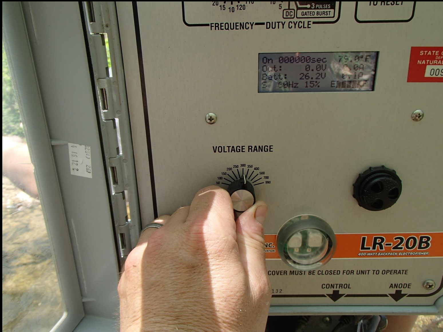
Use of appropriate voltage
