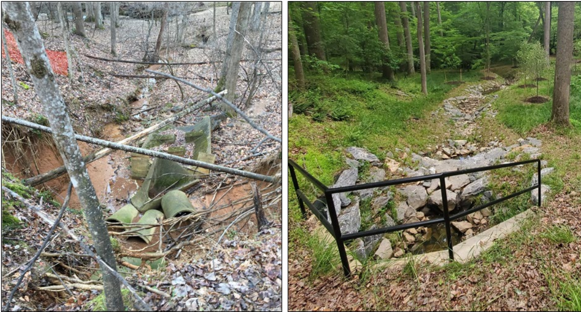
Before and after photographs of a storm drain outfall channel restoration completed 2021 in Watts Branch SVU 3. Photos by Jacqueline Hoban.
