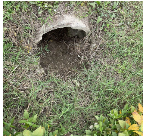
This is a photo of erosion near a culvert.
