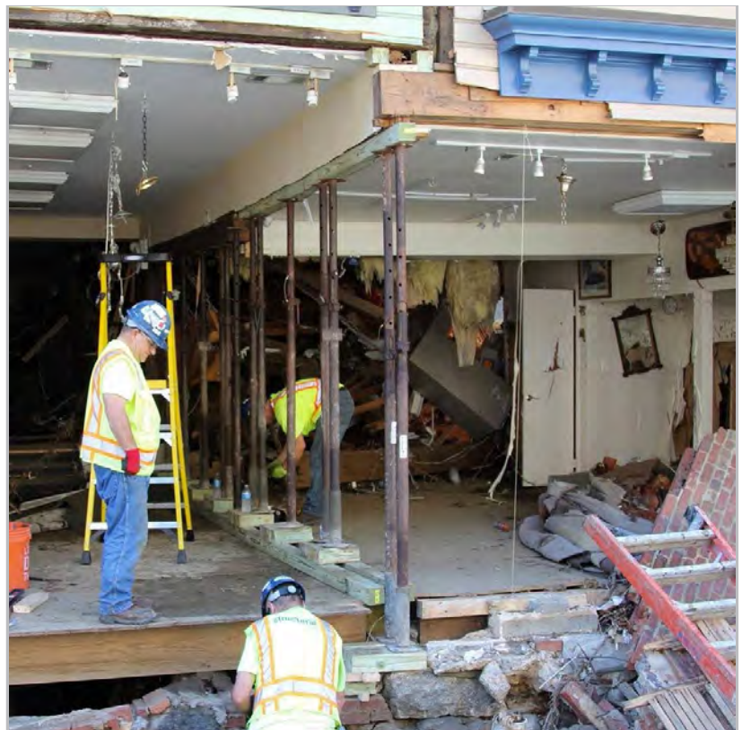
Figure 2.24 - Stabilizing buildings in Ellicott City, Howard County, 2016. (Source: Preservation Maryland)
