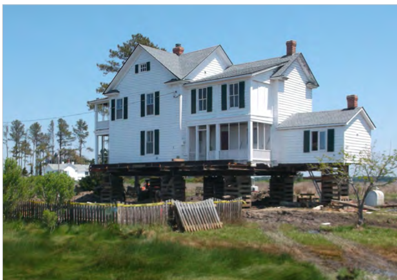
Figure 2.40 - Elevation in progress of a late 19th century historic home on St. George Island, St. Mary's County. The building was elevated to the BFE plus three feet of freeboard. (Source: MEMA)
