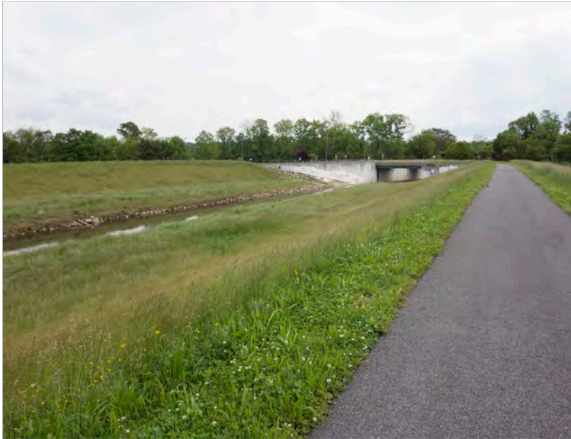
Figure 2.32 - A walking and bicycle path is located on top of the levee in North Brentwood, Prince George's County, which provides protection for the adjacent National Register Historic District.
