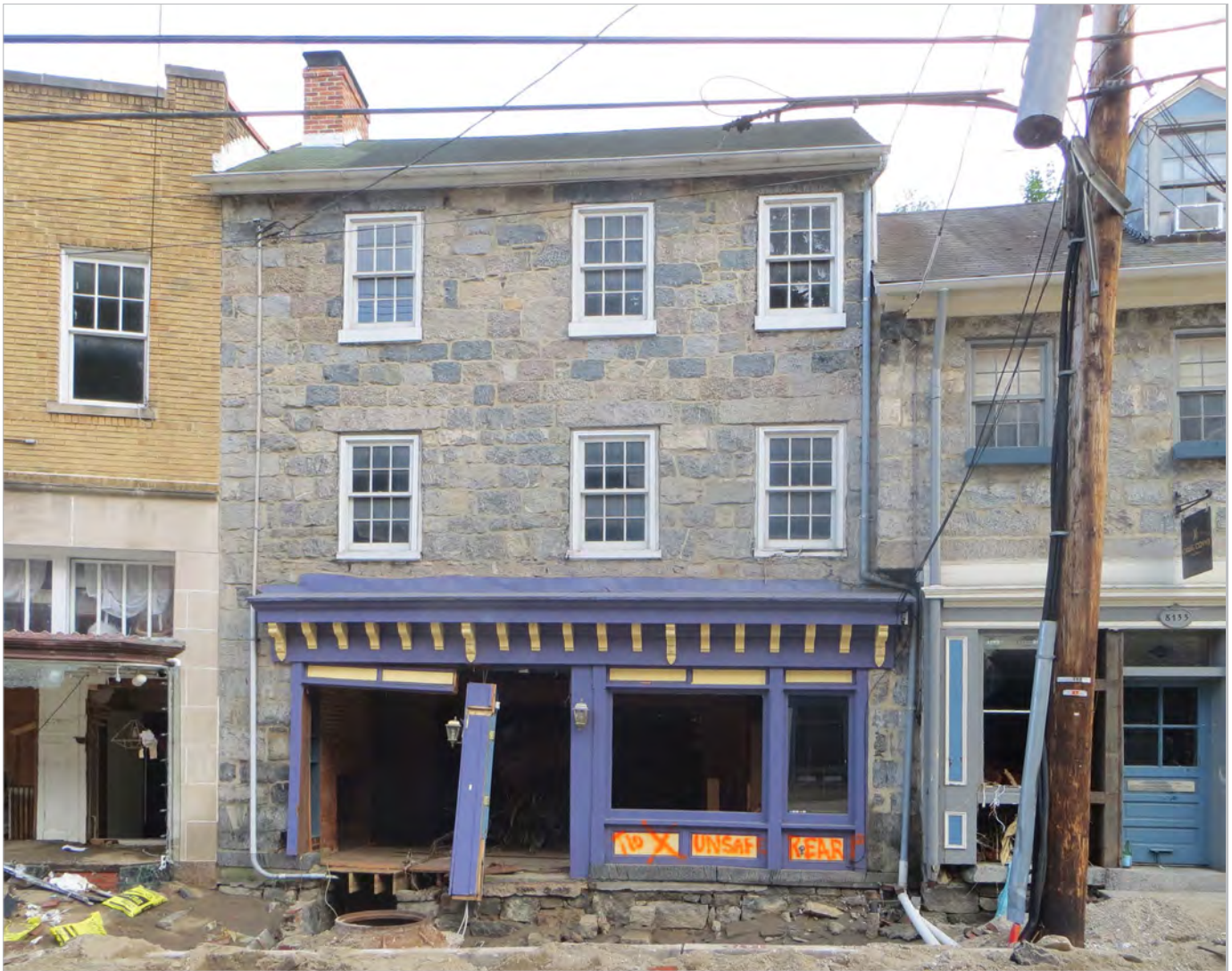
Figure 2.21 - Building Tagged as "Unsafe Rear" by first responders. The rear wall of the first floor was blown out due to floodwater entering the front of the building. Ellicott City, Howard County, 2016
