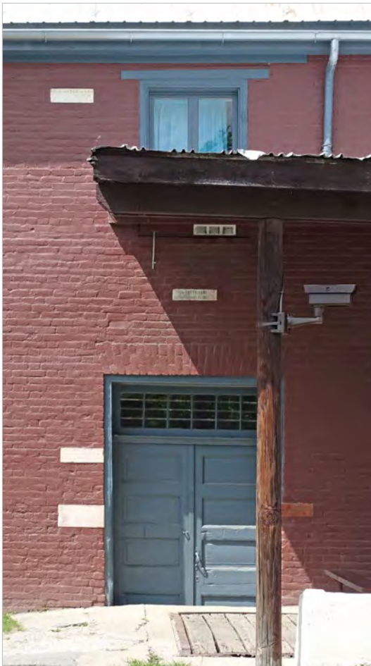
Figure 2.14 - Chesapeake & Ohio Canal Cushwa Warehouse (constructed circa 1790 – 1810) located at the canal’s edge has historical high watermarks visible in white block on the face of the building noting the depth of flooding from five food events from the mid-19th to early 20th century. Williamsport, Washington County.
