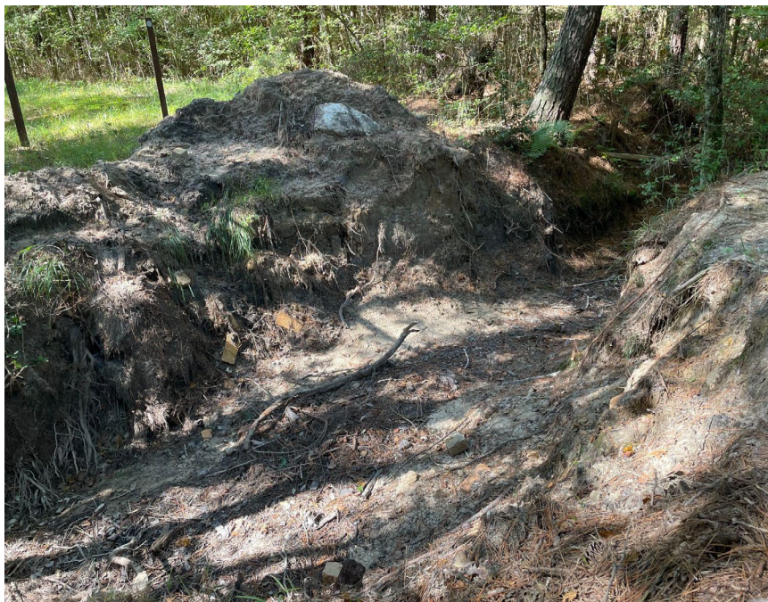
This shows how much erosion can occur when a water control structure is damaged.
