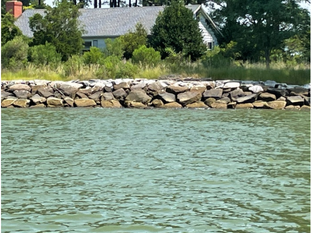
Photo 7 - Shoreline Protected with Revetment
